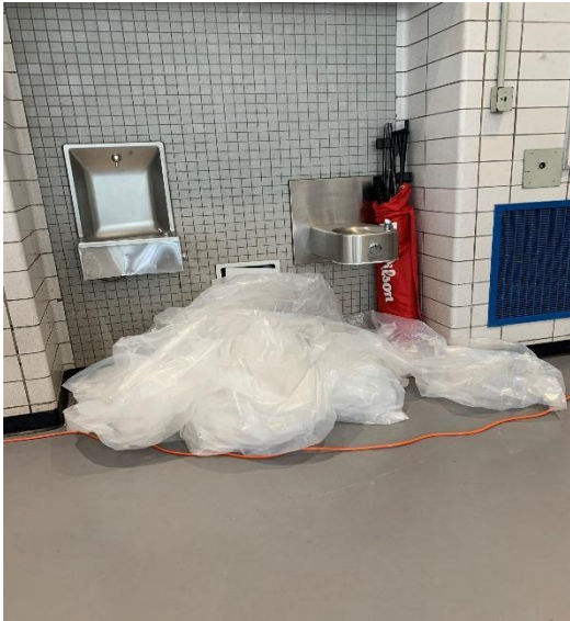
Jackie Robinson College, Manhattan. Plastic and cords are tripping hazards on pathway for those with low vision or those who are blind.
