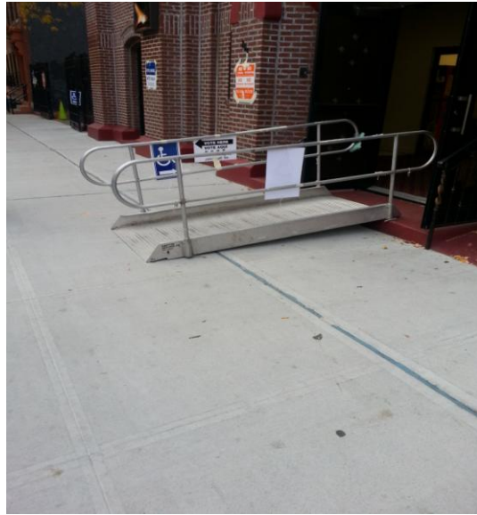
Bethel Baptist Church, Brooklyn - Ramp too small for the space
