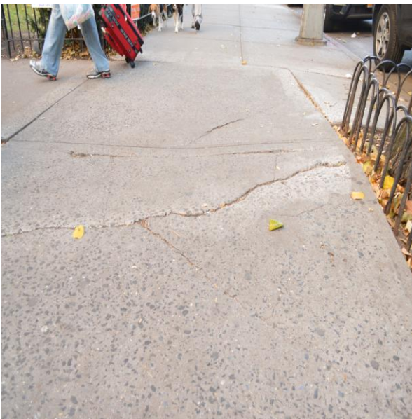
Seward Park II, NY, NY – Extreme crack, uneven sidewalk
