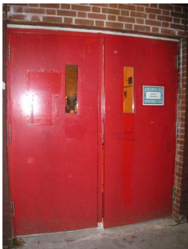
This entrance door at PS 20 (Queens) is heavy and there are no accessible handles. No door monitor was present outside to provide assistance.
