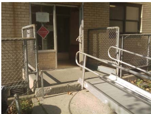
At Masaryk Towers (Manhattan), the front door was left partially opened, obstructing the path from the ramp to the entrance for voters using wheelchairs.
